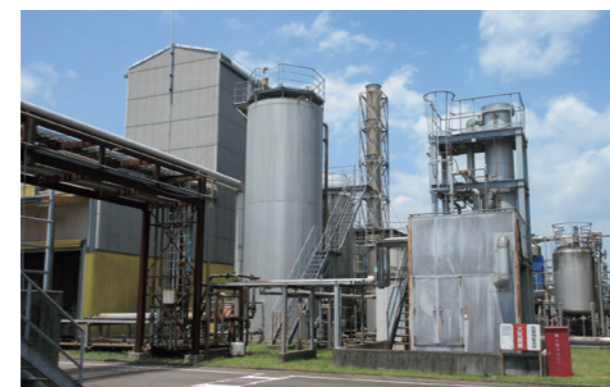
Equipment for converting shochu lees into feed at Kurokabegura
