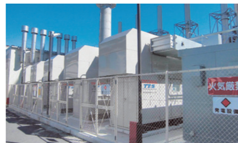
Micro gas turbine co-generation system
